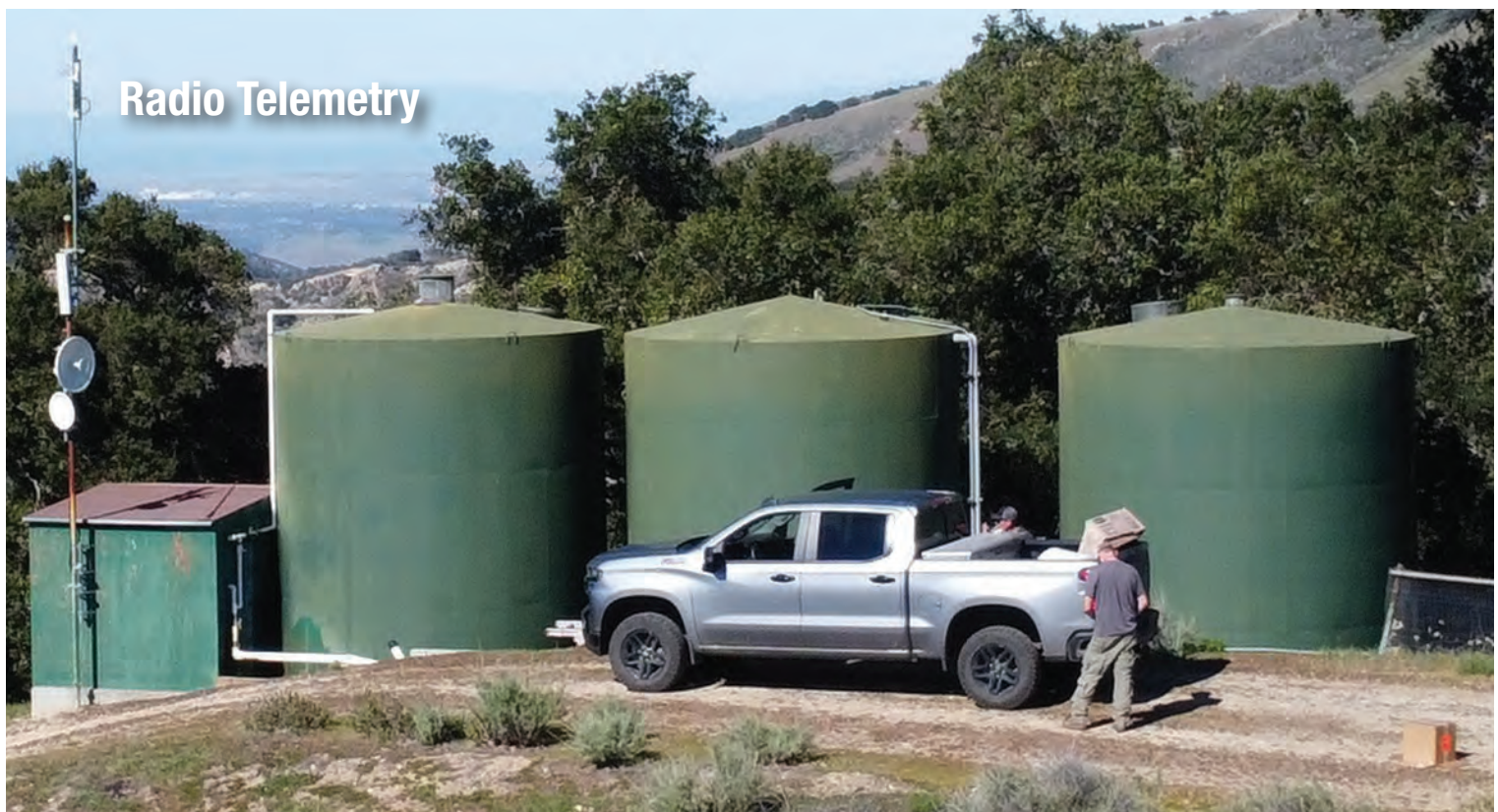
Potable Water and Fire Storage
