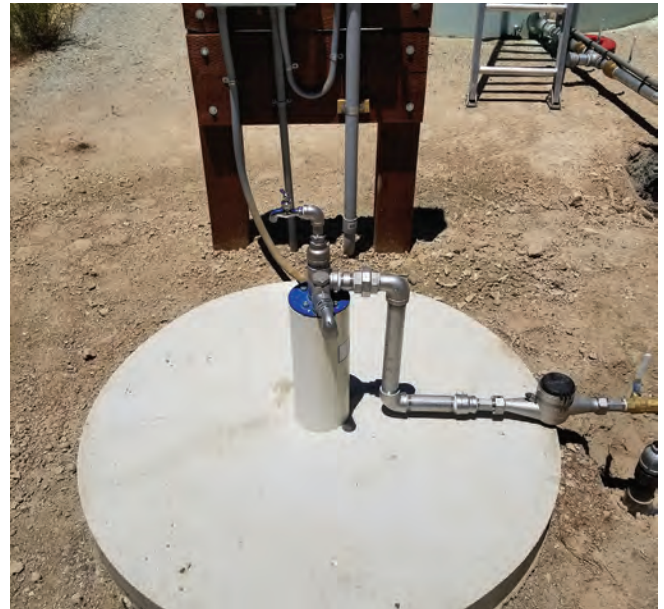
Groundwater Well Submersible Pump
